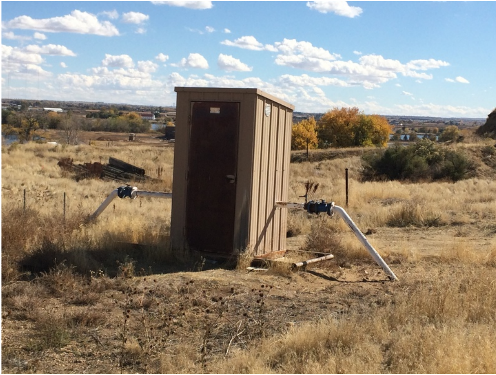
Texas Tea meter shed
