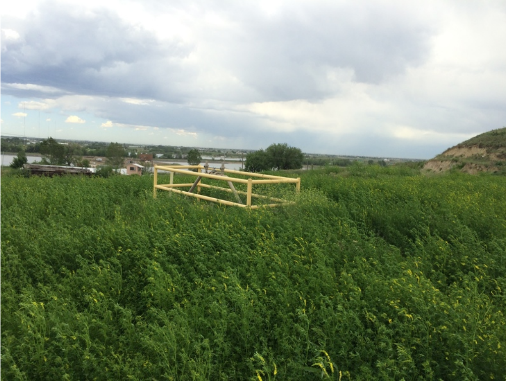
Anadarko 3" Pipeline Riser
