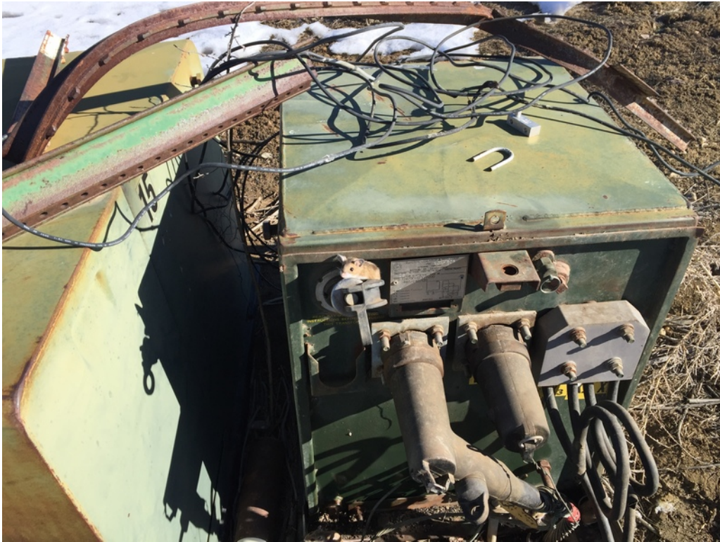
Two Texas Tea electrical transformers
